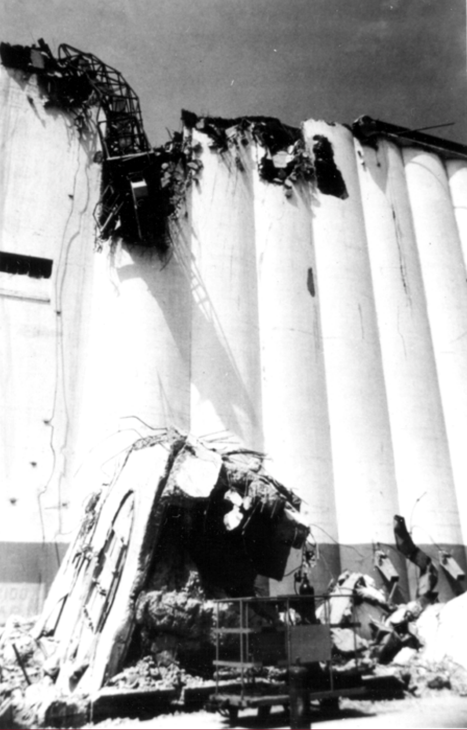
Peru Earthquake October 3, 1974. This grain elevator complex in the port of Callao partially collapsed. 1974. Page 7, Earthquake Information Bulletin, v.7, no.2. Bulletin-0007
