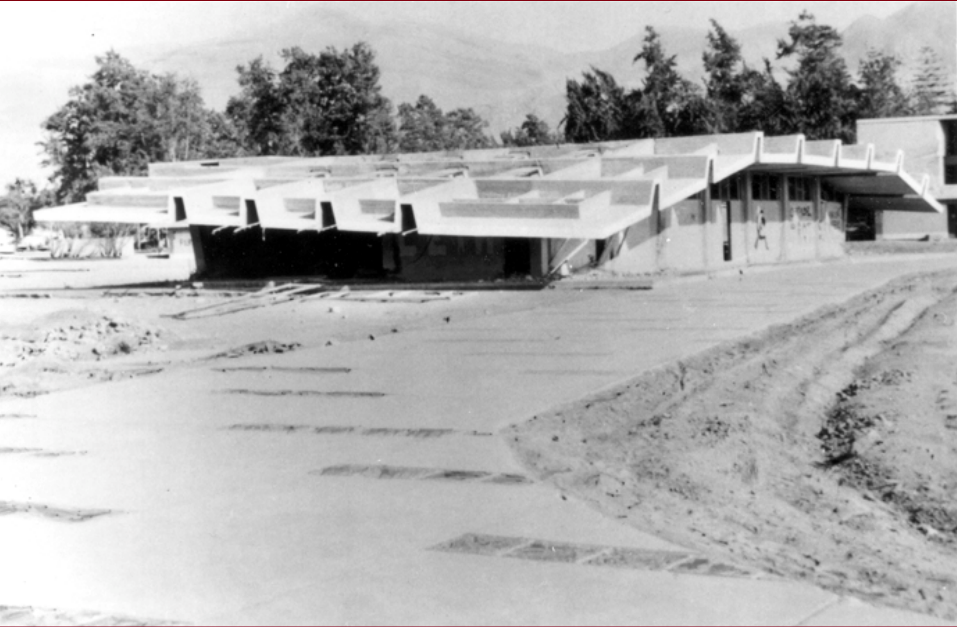
Peru Earthquake October 3, 1974. Example of the extensive damage in La Molina District. This classroom and a laboratory building at the Agrarian University partially collapsed. 1974. Pages 6-7, Earthquake Information Bulletin, v.7, no.2. Bulletin-0007
